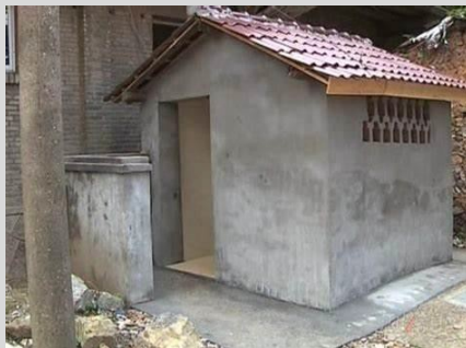
Typical dry latrine in northern China
