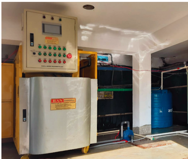
FIGURE 07: Electrochemical Reactor. Source: RAN Corporation.
