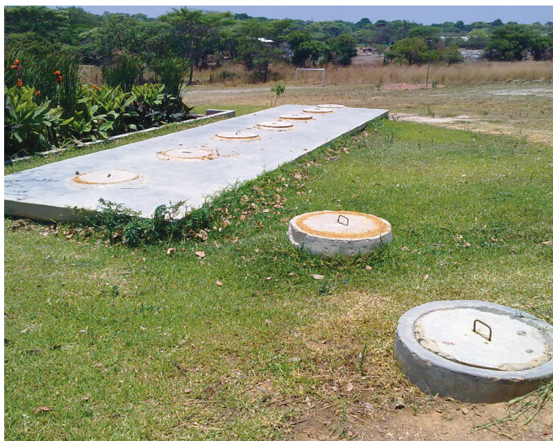
FIGURE 03: Installed ABR with manholes for each of the 6 chambers. Source: Gates Open Research, UPM, Anaerobic Baffled Reactor (ABR) Design Considerations for Faecal Sludge.
