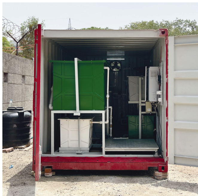
FIGURE 10: Containerized NEWgenerator system. Source: Documentation by UPM GmbH team during a visit to Elefo, 2022.
