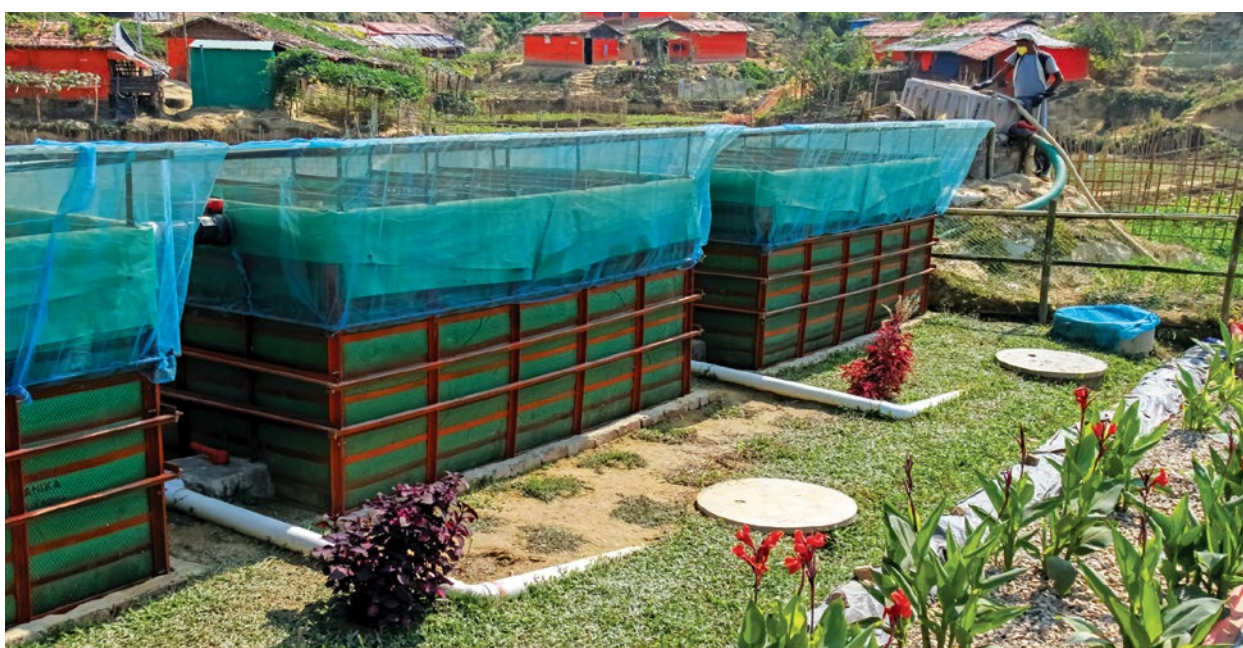
Figure 3: FSTP unit of Practical Action in a Rohingya camp
