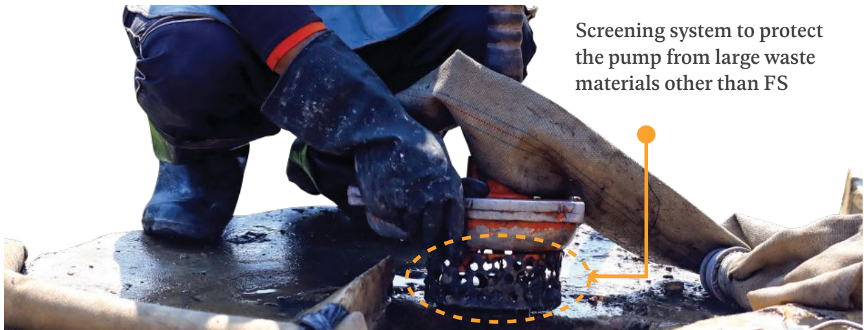
Figure 6: Screening system at the pumping chamber of the hi-cap sucker
