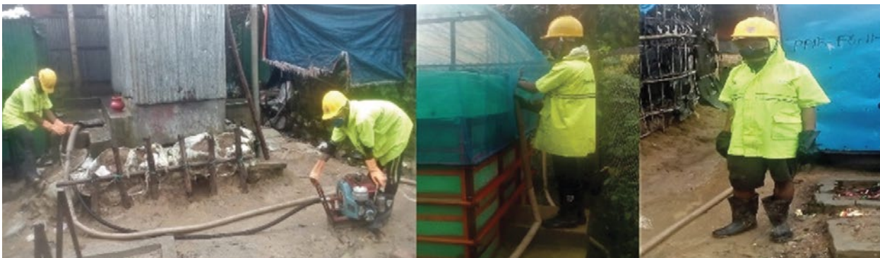
Figure 23: Two sanitation workers operating the hi-cap sucker machine to collect FS from containment (left), one worker dumping FS into solid-liquid separation unit (middle), one worker looking after sludge collection pipe (right)
